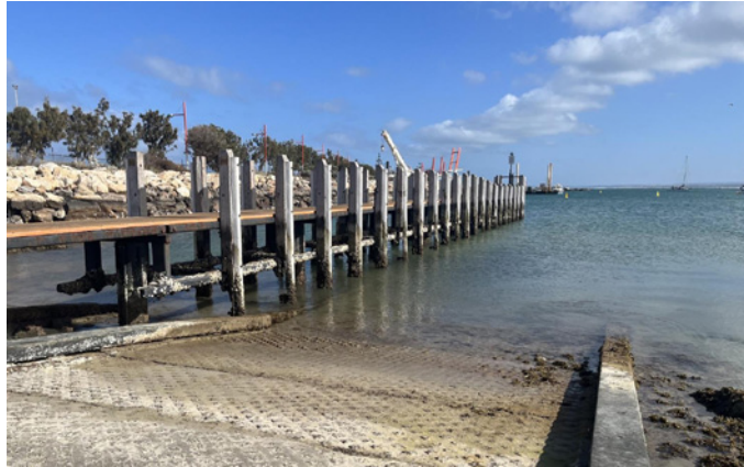
Looking good: Repair work in progress at Geraldton’s Francis Street finger jetty. PIC: City of Greater Geraldton
